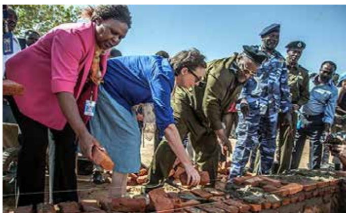
On 5 December 2017, UNAMID's Rule of Law Section, in partnership with the Government of Canada, supported the construction of a dormitory, a child-friendly space and a visitors' bay for women inmates in Kutum prison, North Darfur. The project is part of the Mission's continued efforts to strengthen the rule of law across Darfur. Photo by Mohamad Almahady, UNAMID.
