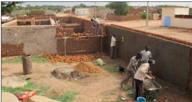
On 26 July, in Nyala, South Darfur, UNAMID launched the renovation of Alwuhda Youth Centre. The project is part of a programme to benefit at-risk youths in Darfur. Photo by Saeed Abdalla, UNAMID.
