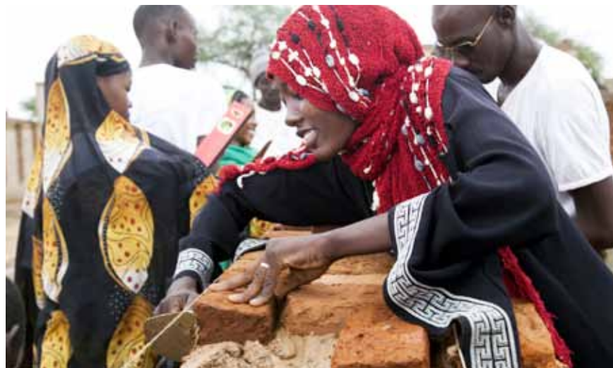
On 15 August 2012 in Althoura Shemal, North Darfur, young men and woman work to build a community centre in one of UNAMID’s community-based, labour-intensive projects (CLIPs). This project, facilitated by UNAMID’s Disarmament, Demobilisation and Reintegration section, provided vocational training to 80 young people. Photo by Albert González Farran, UNAMID.
