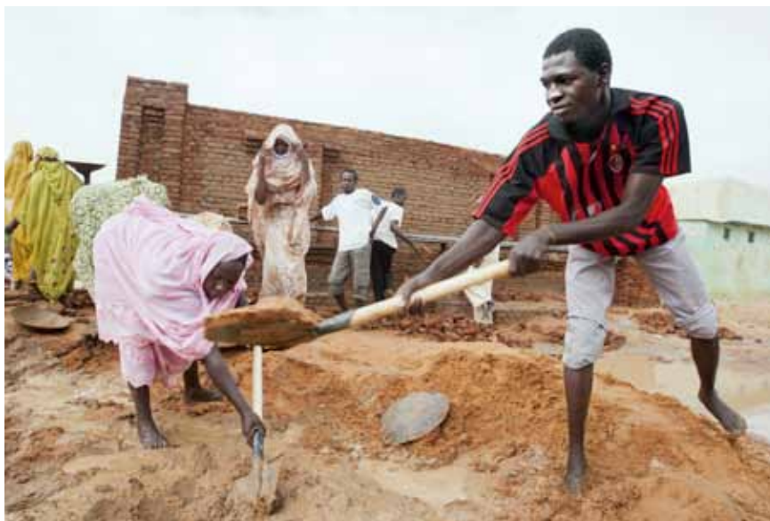
On 7 October 2012 in Althoura Shemal, young men work to complete a community centre in one of UNAMID’s community-based, labour-intensive projects (CLIPs). Photo by Sojoud Elgarrai, UNAMID.
