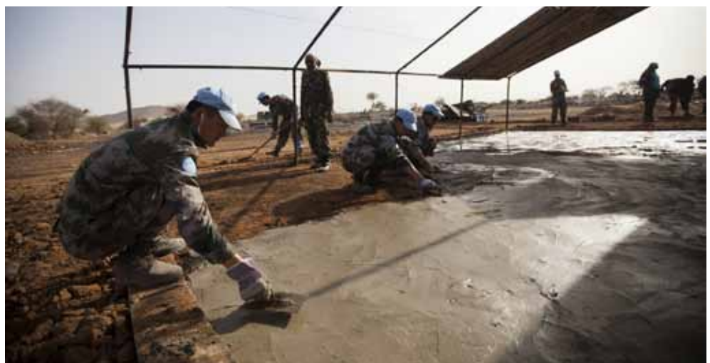
On 7 April 2014 in Khor Abeche, South Darfur, UNAMID engineers work to build a community centre for displaced people who had sought refuge in the Mission's camp. The community centre, one of two, is located inside a secure 70,000 square metre area that the Mission set up for the Darfuris who took refuge inside UNAMID's premises. Photo by Albert González Farran, UNAMID.
